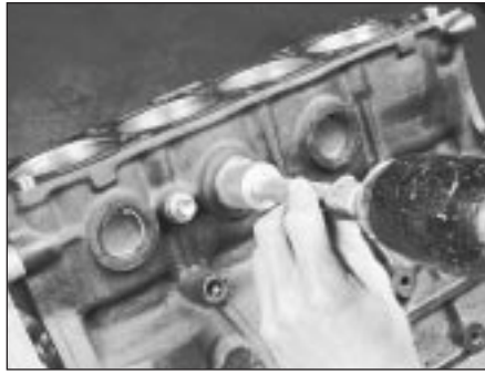
11.9 A large socket on an extension can be used to drive the new core plugs into their bores
